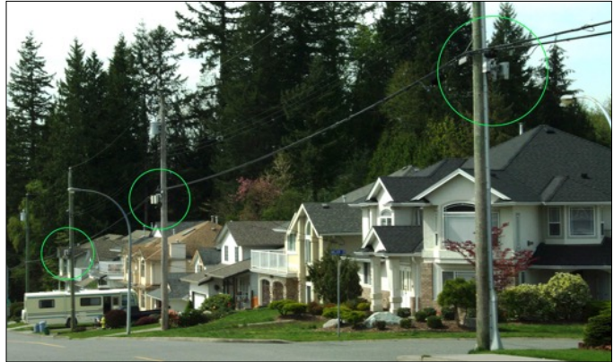
Wireless transmitters in a residential neighborhood
