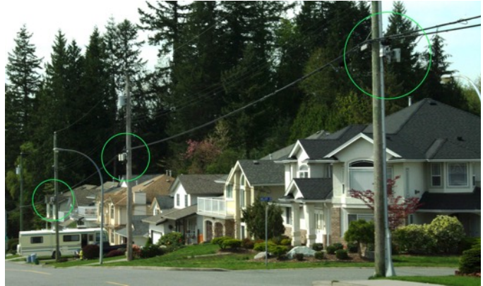
5G transmitters on residential poles in California
